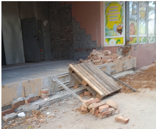
I’m sure this is OSHA compliant, right?
